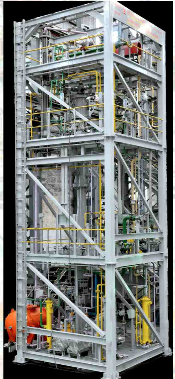
Skid mounted unit
